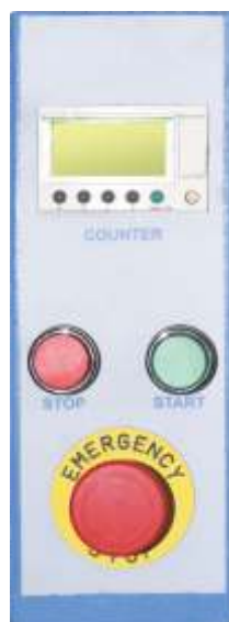
Control Box (Close-up)
